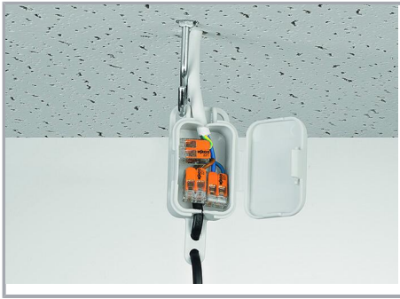
Pendant light connection in a suspended ceiling
