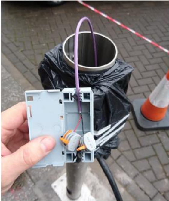
Figure 2 - Wago connectors linking up the serial bus
