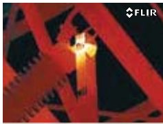
Incorrectly secured connection
